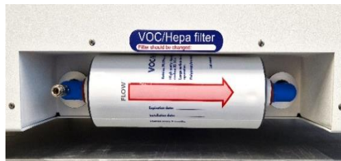
Figura 12.3 Filtru COV/HEPA corect instalat
